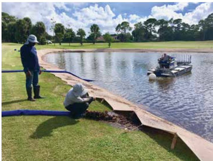
Shallow pond sediment is pumped with our amphibious work boat directly into the SOX containment system to restore the shoreline.
