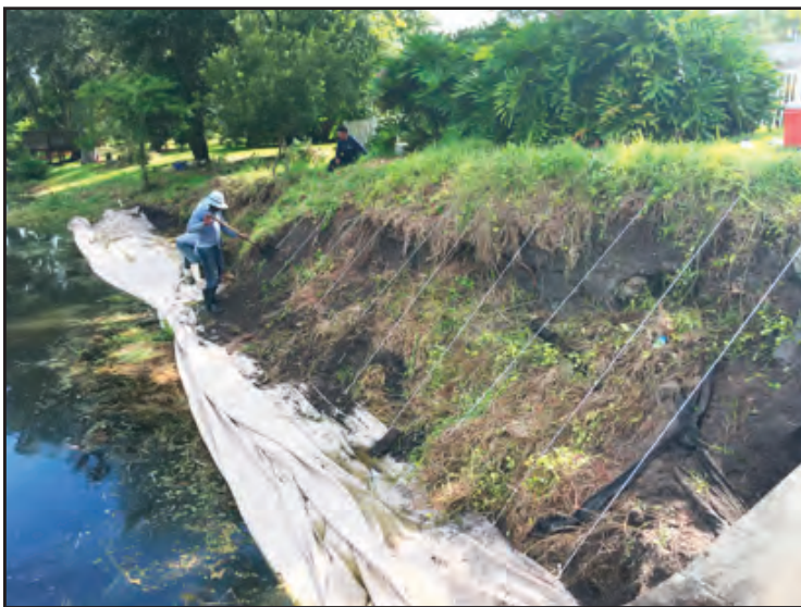
The SOX System is put into place while the canal bank is prepped and our patented anchoring and channeling system is secured to solid ground.
